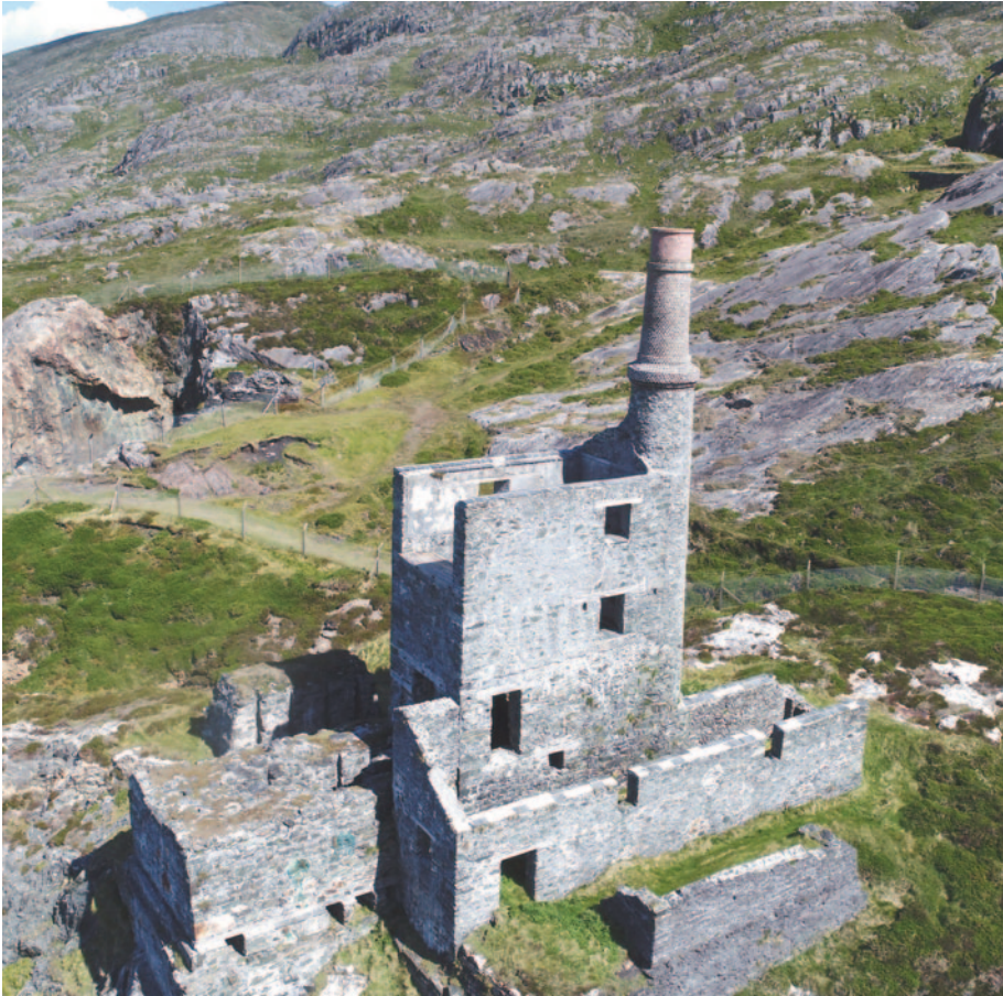
Fig. 4. 'Man engine house' of 1862, at Allihies, county Cork, after conservation by Mining Heritage Trust of Ireland.
