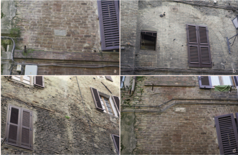
Fig. 6. Examples of anti-seismic repairs documented during the archaeo-seismological analysis: bond stones (11a and 11d) and relieving arch (11b and 11c).
